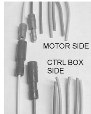
Signal cables with bullet crimp terminals
